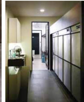
ABOVE: As the Ladrang kitchen is set to cater for both the Ladrang staff and many guests, it has been fully equipped with industrial-sized refrigerators, freezers and extensive cooking facilities.
